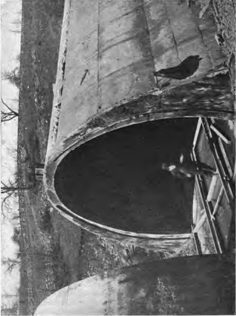
PLATE 74.—Contract 11. Cut-and-cover Arch. This section was cast between steel forms with steel plates in expansion joints at 60-foot intervals. Steel plates 6" X 3" were placed in both invert and arch joints to act as water stops.
